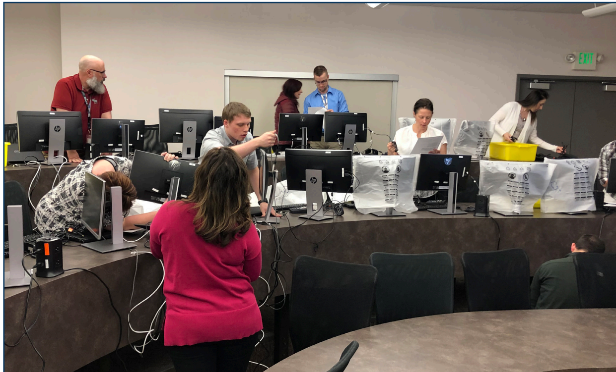
Jeffcom employees set up the backup center
